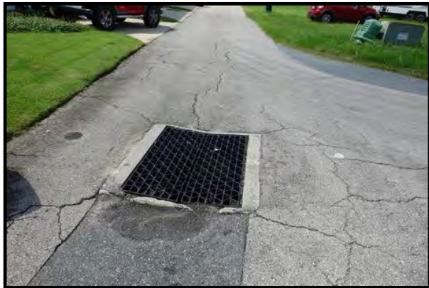
Figure 1 – Stormwater Catch Basin
