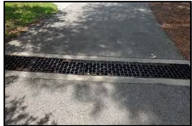
Figure 2 - Stormwater Catch Basin
