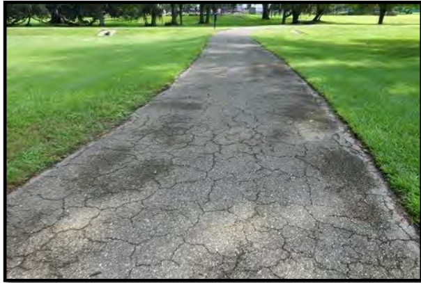
Figure 1 – Significant Alligator Cracking
