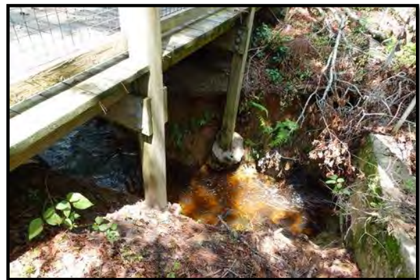
Figure 4 - Bridge 5 Column Undermined
